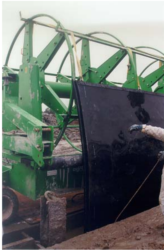
Insertion prior to reaching the desired depth - The straps which were used for rolling up the panel are used for hanging the liners afterwards.
