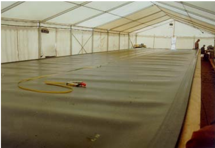
Prefabrication of the HDPE panels (AGRU HDPE liner + 2 AgruLock profiles) in a welding tent to maintain steady welding conditions
