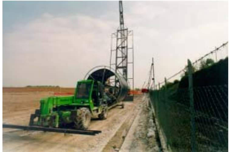
Concrete boundary of the trench - the installation frame in the background, the installation drum in the foreground
