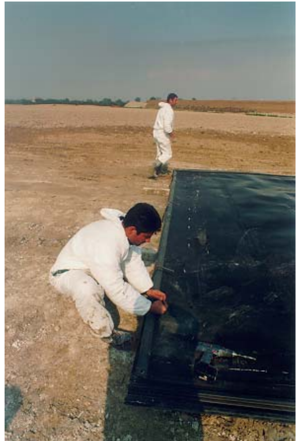
Clamping of the HDPE panel with steel bars over the whole panel width
